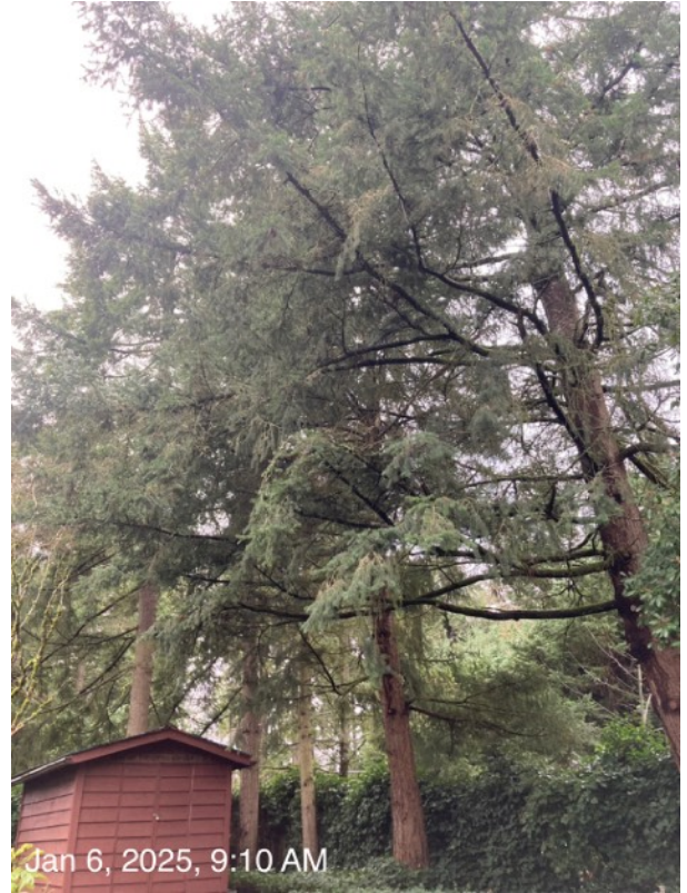
Trees #21-#25 noted as healthy and vigorous. Shed foundation damage noted caused by soil displacement from root growth.
