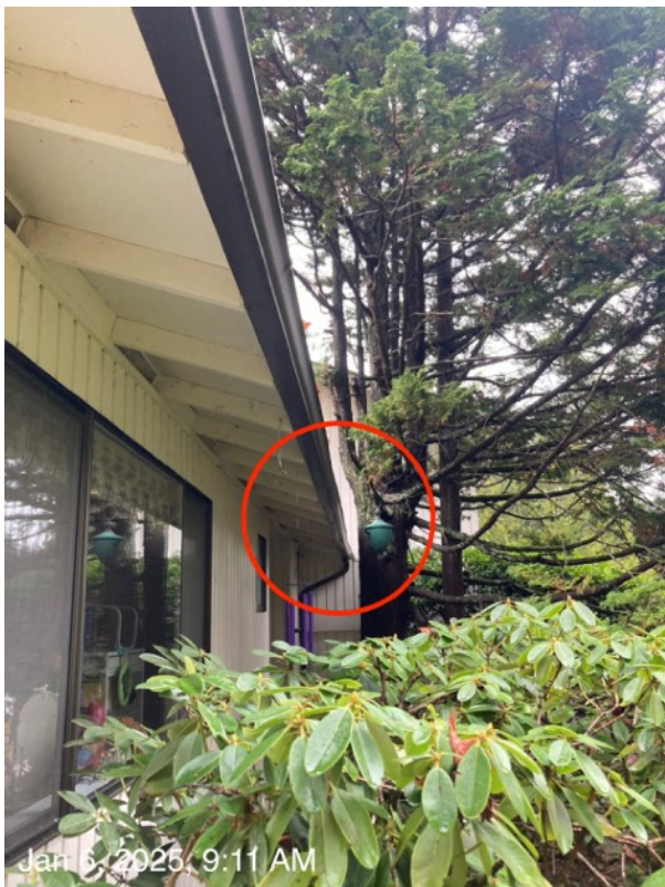
Tree #3 in extreme proximity with home.
